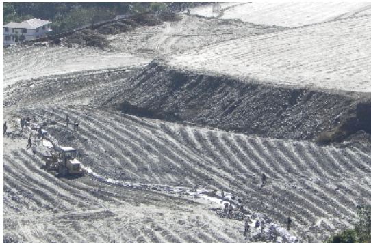
Damage due to deforestation and urbanisation
